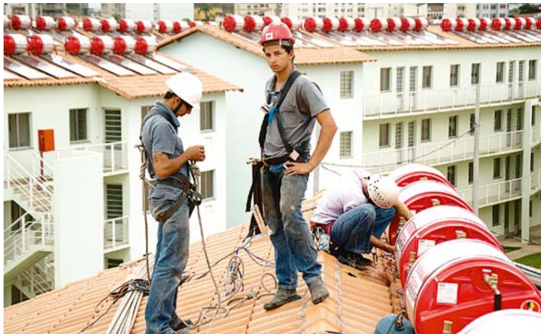
Installation of gravity systems as part of the Brazilian “Minha Casa Minha Vida” project. The tank holds 200 L and the collector area is approx. 2 m 2 .
